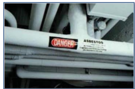
Good Practice: Asbestos-coated pipes are properly marked.
