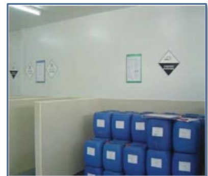
Good Practice: Proper signs and labels.
