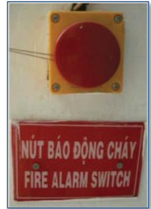
Good practice: Fire alarm switch in native language
