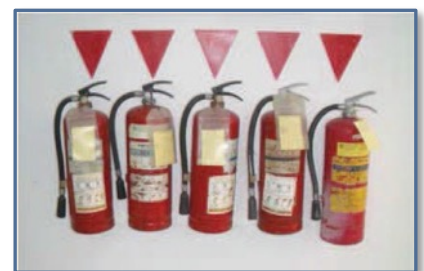
Good practice: Fire extinguisher types for potential hazards are provided and tagged
