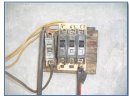
(IA) Circuit breaker with exposed and damaged wiring! Circuit breakers must be labeled and enclosed.
