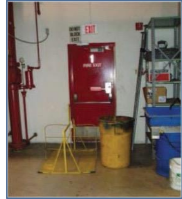
Bad Practice (IA): Fire exit is blocked by trash container and equipment
