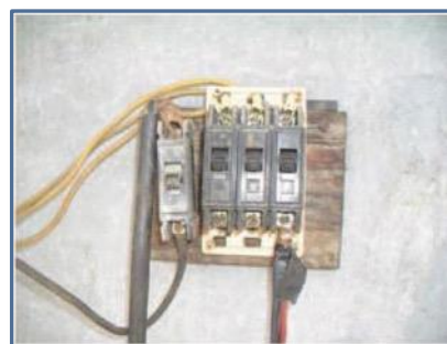
(IA) Circuit breaker with exposed and damaged wiring! Circuit breakers must be labeled and enclosed.
