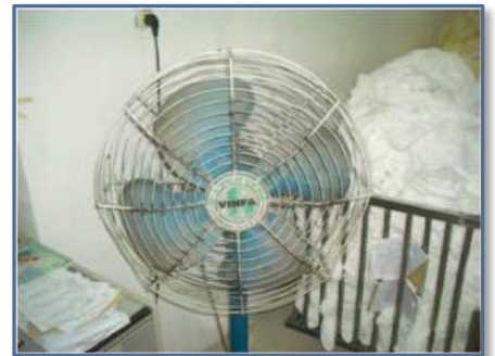
Good Practice: Typical fan used to cool workspace.
