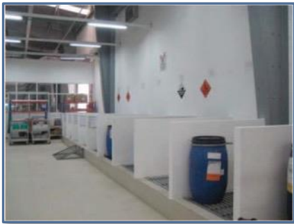
Good Practice: Secondary storage is segregated and well lighted.
