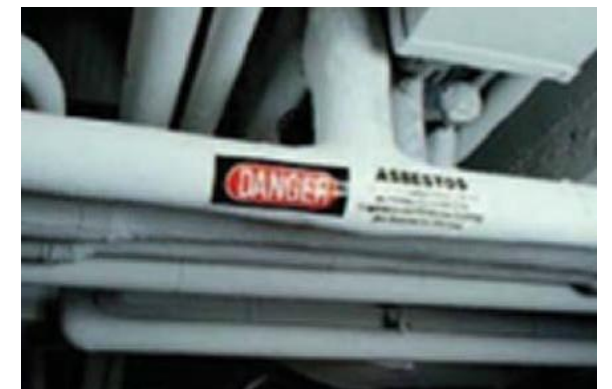
Good Practice: Asbestos-coated pipes are properly marked.
