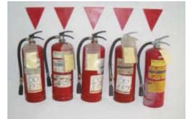
Good practice: Fire extinguisher types for potential hazards are provided and tagged
