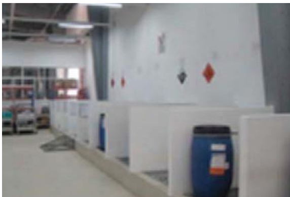
Good Practice: Secondary storage is segregated and well lighted.
