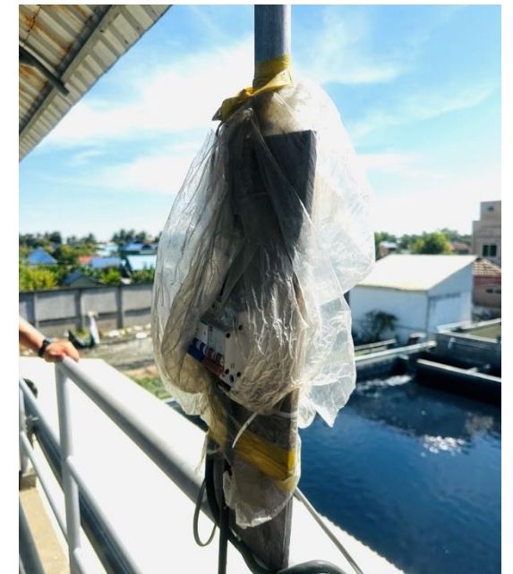
IA Circuit breaker with exposed and damaged wiring! Circuit breakers must be labeled and enclosed.
